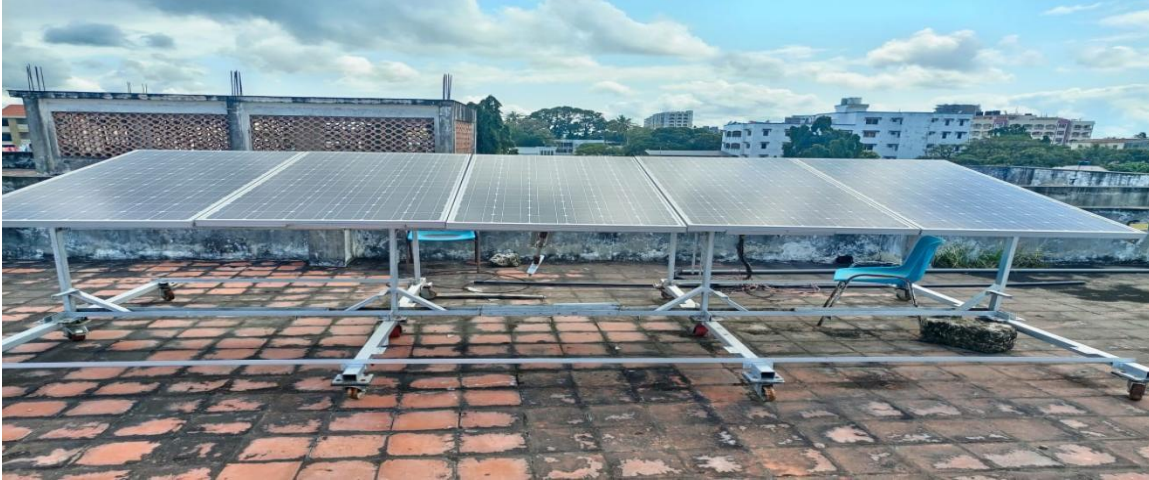
Figure 3. Photos of roof-top solar PV mounted on top of the Renewable Energy Laboratory building at Technical University of Mombasa, Kenya
